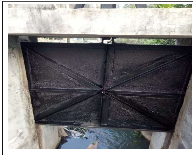
HALISAHAR DRAIN LOCKGATE
